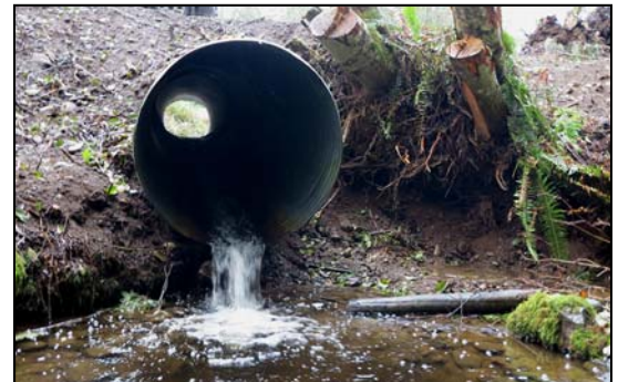
Before: Undersized culvert blocked fish passage.
