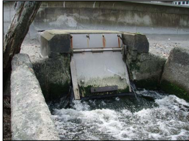
Figure 24 - tide gate at mouth of Cooper Creek (existing configuration)
