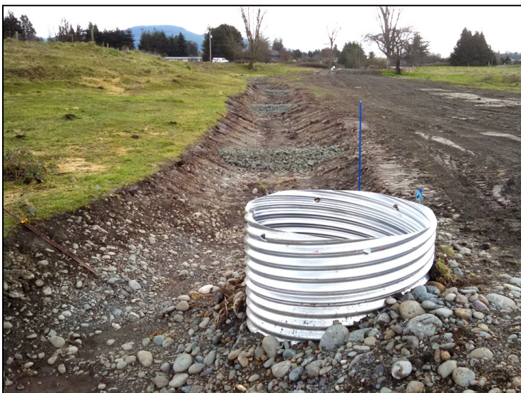
View of infiltration trench looking upstream toward McComb Road. New irrigation pipeline was installed to the right.
